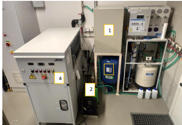
Figure 3. Water treatment unit
